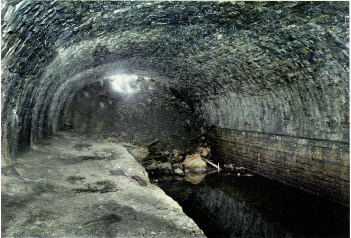
The infilled west portal of the second canal tunnel at Rain Hall quarry. Photo Nick Catford
